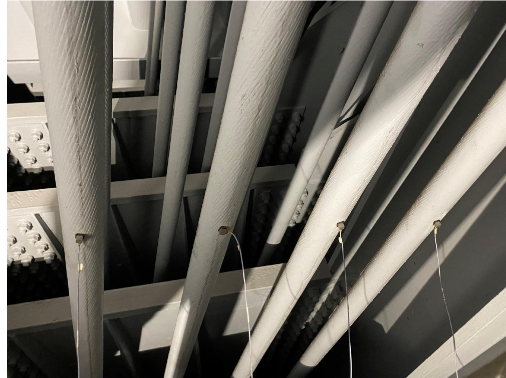
ACCELEROMETERS on ROPES
